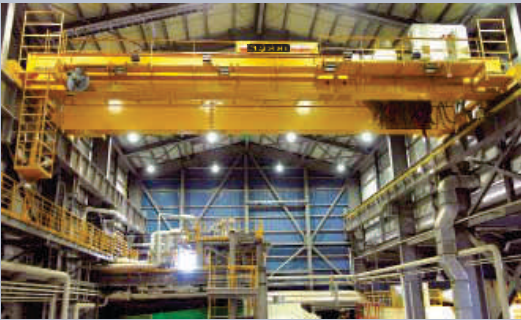
87T Power station crane
