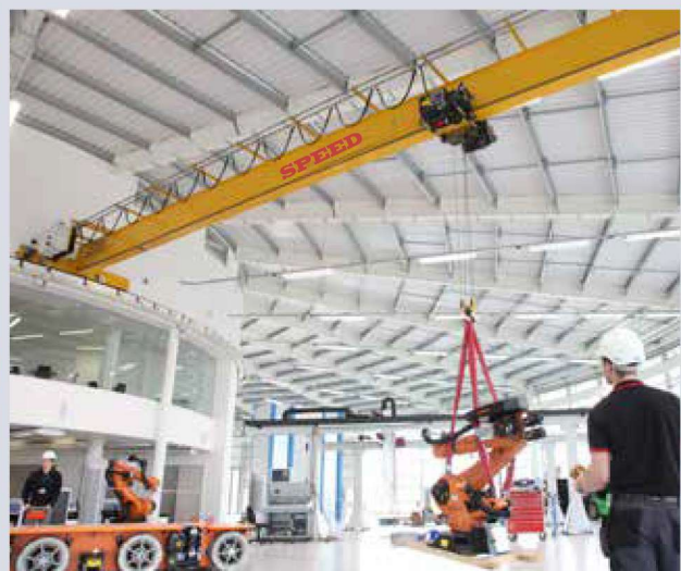
SDWH cranes forms an essential part of operations in this iconic circular factory.
